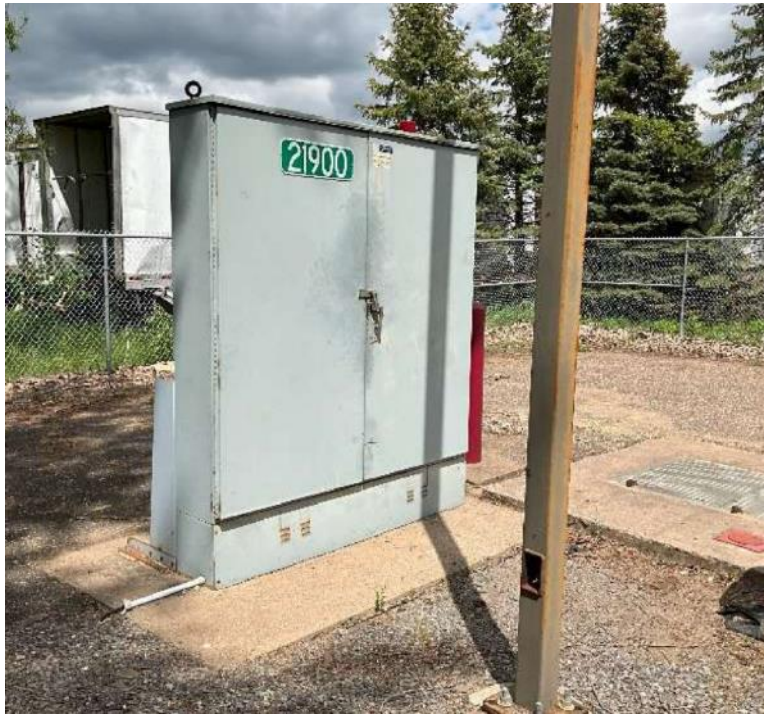
Figure 2.5: Lift Station No. 3 (137th Ave.) Control Panel Enclosure
