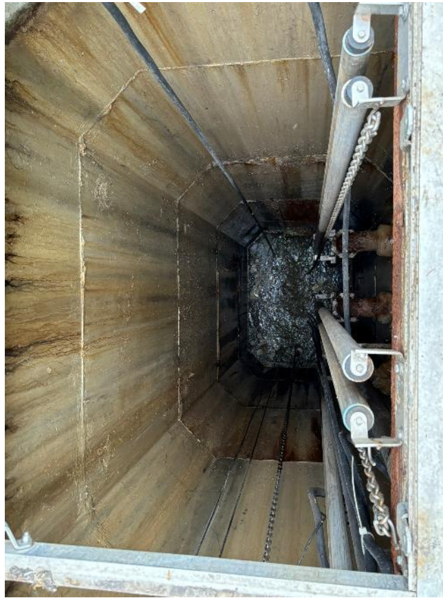
Figure 2.1: Lift Station No. 3 (137 th Ave.) Wet Well
