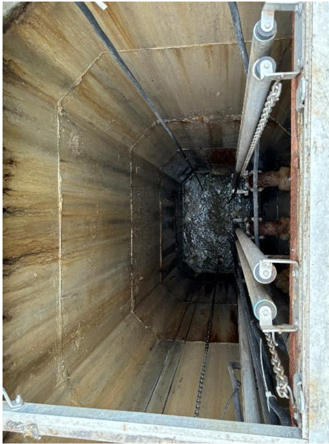
Figure 2.1: Lift Station No. 3 (137 th Ave.) Wet Well
