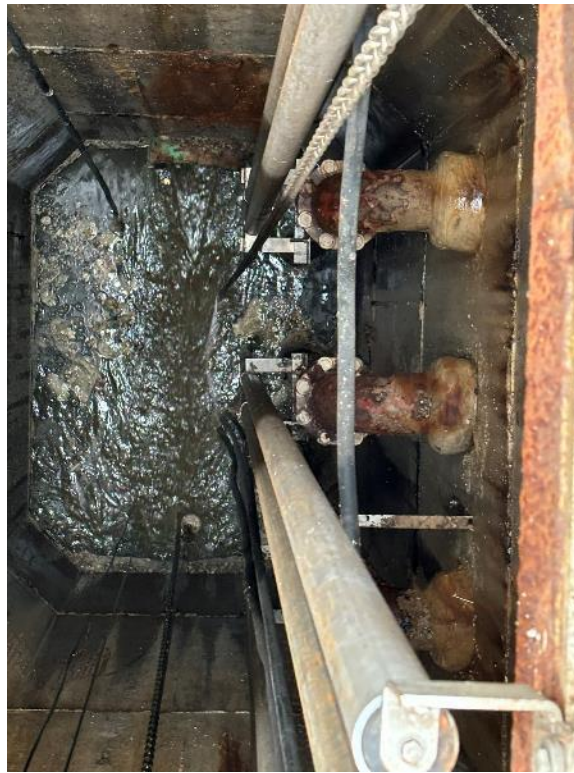
Figure 2.3: Lift Station No. 3 (137th Ave.) Wet Well
