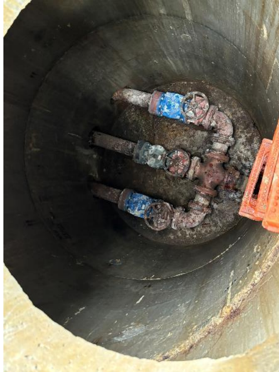
Figure 2.4: Lift Station No. 3 (137th Ave.) Valve Vault
