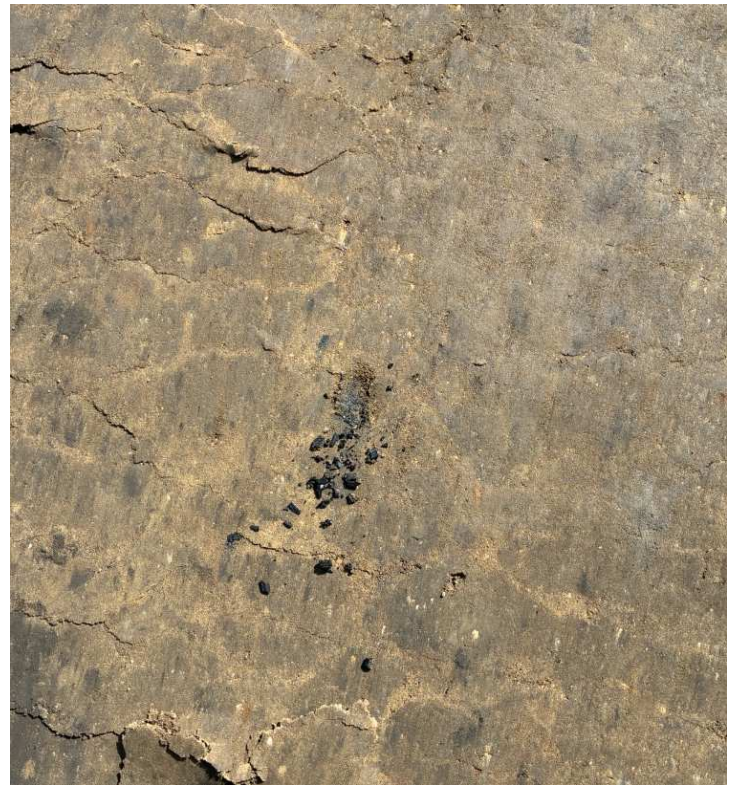
6-15-26 - Asphalt contaminates located during correction
