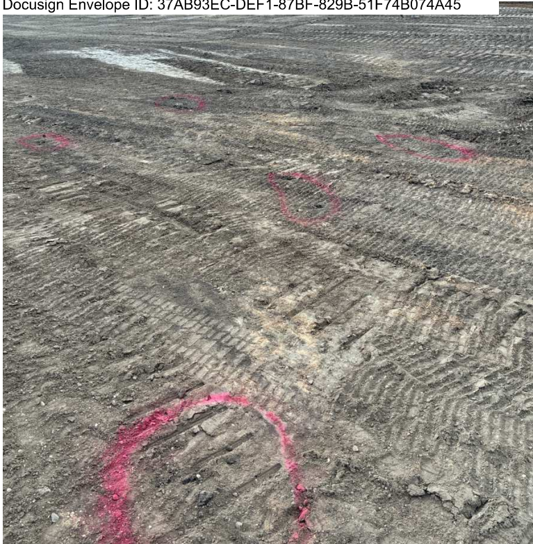
6-10-26 - Asphalt contaminates located during correction
