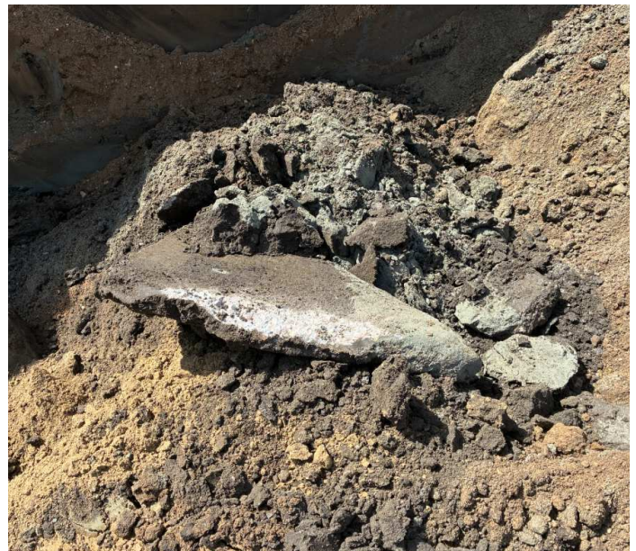
6-15-26 - Construction debris removed from soil
