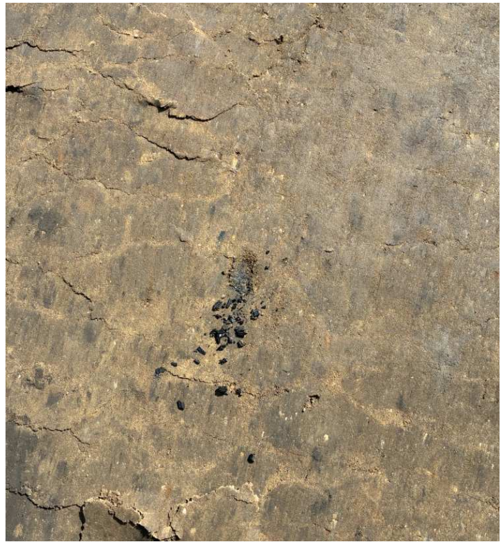
6-15-26 - Asphalt contaminates located during correction
