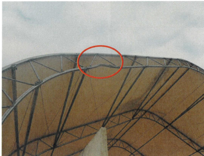
Figure 3. Bent bottom chord of truss on east elevation.
