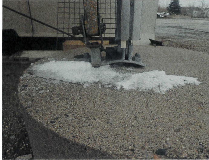
Figure 4. Bent base plate of first truss on east elevation.
